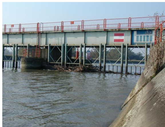
Fig. 6 Probe protection pipe on the bank— clogging of coarse rack
