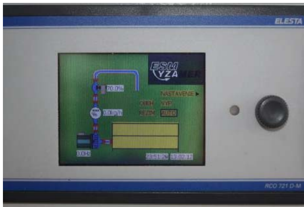
Figure 2 Control system panel in the door of switchboard [Photo by authors]
