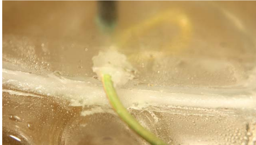
Fig. 6 Silicone sealant partly degraded by chlorine (originally transparent) [Photo: R. Kuracina]
